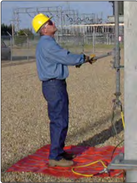
Operate Switches Safely
