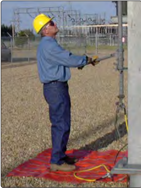
Operate Switches Safely
