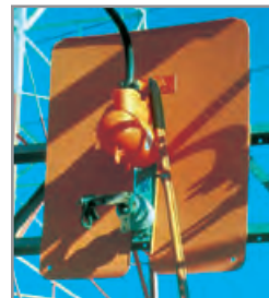
Barrier and Switch Jaw Guard installed on a Substation Switch.
