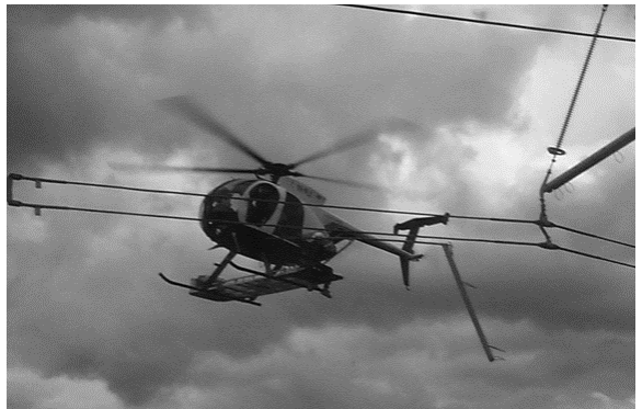
Removal by helicopter, of the shroud from composite insulators prior to energising
