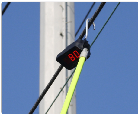
DVI-500T Digital Voltage Indicator In Use
