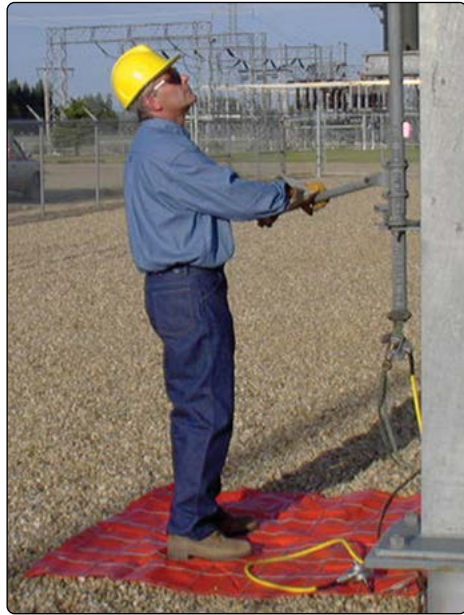
Operate Switches Safely
