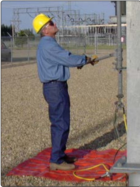
Operate Switches Safely
